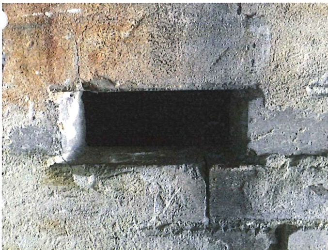
Photo 7 - Deteriorated section of internal wall
