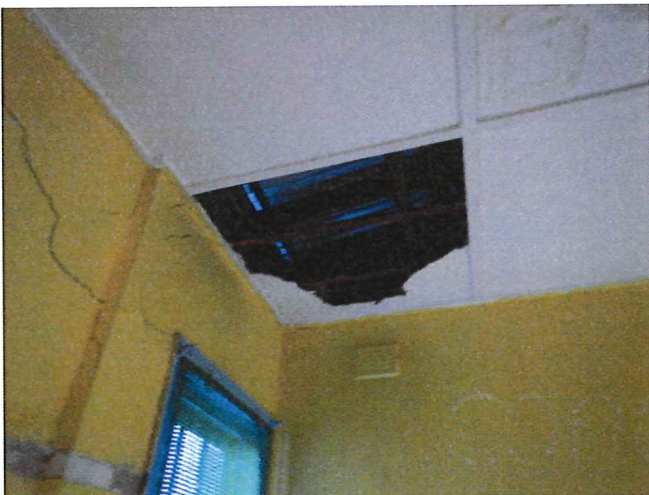
Photo 31 - Damage to roof of upper level apartment
