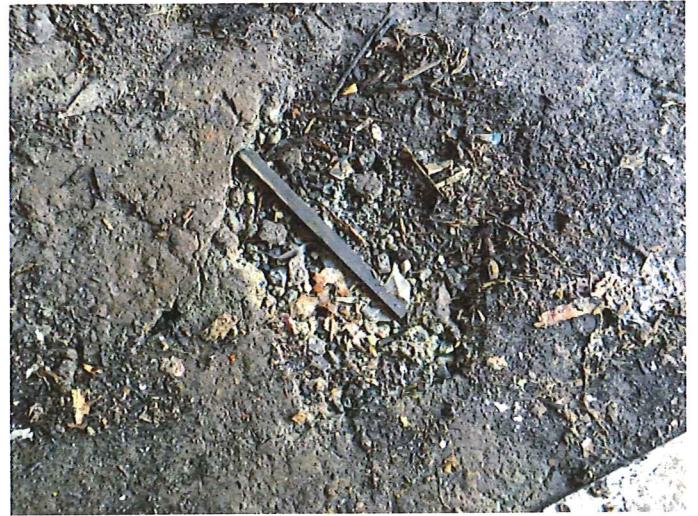
Photo 18 - Damage to ground floor slab
