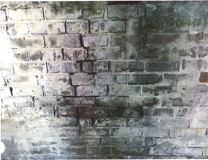
Photo 9 - Deteriorated section of internal wall
