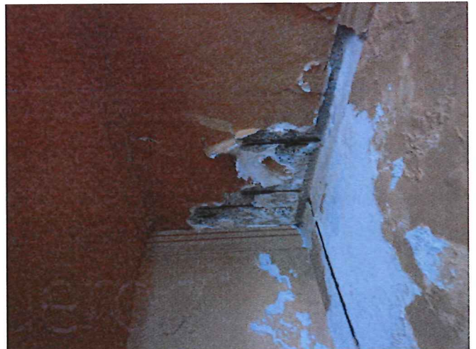
Photo 32 - Damage to roof of upper level apartment
