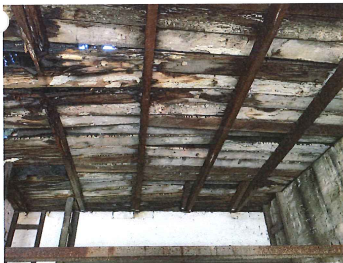
Photo 19 - Significant damage to roof
